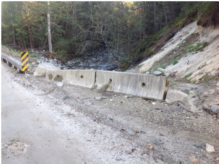
concrete barriers on left bank are backwards
