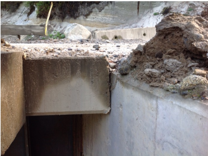
left bank ballast wall hung 50mm lower than deck panel - probe to grader damage
